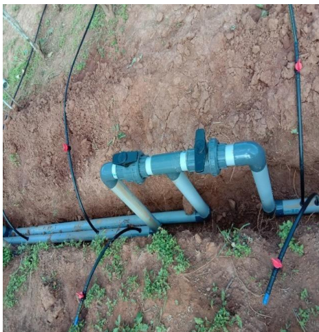
Water control valves
