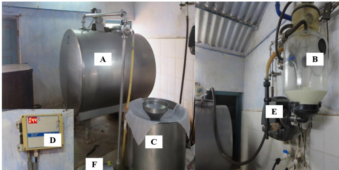
A : Bulk milk cooler (BMC) D : Temperature display for BMC B : Buffer tank for machine milking E : Milk transfer pump from buffer tank to BMC C : Balance tank for manual milking F : Milk transfer pump from balance tank to BMC
