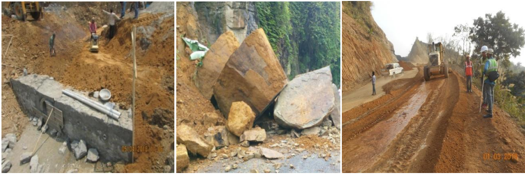
Fig. 8. Some pipeline works under progress of NH in Mizoram (Courtesy: Er. J. Nayak, BBSR)
