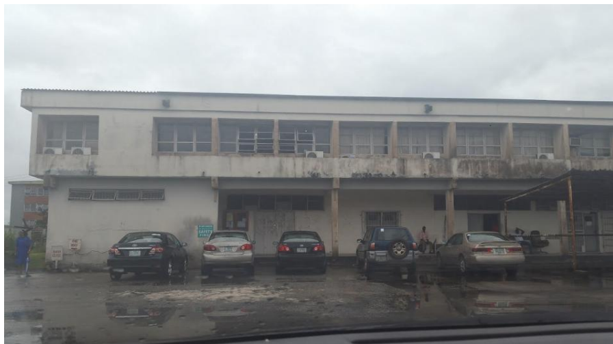
Plate 3. Defective plastering and rendering
