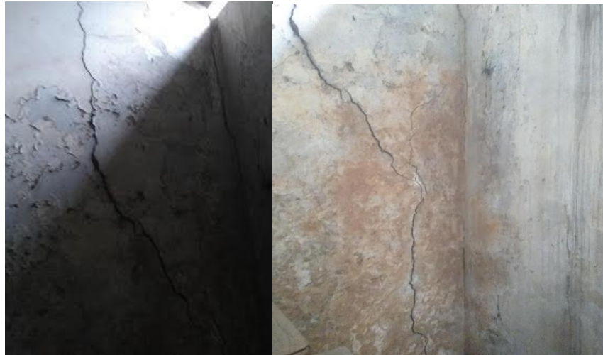
Plate 1. Cracks as a result of the settlement of the foundation
